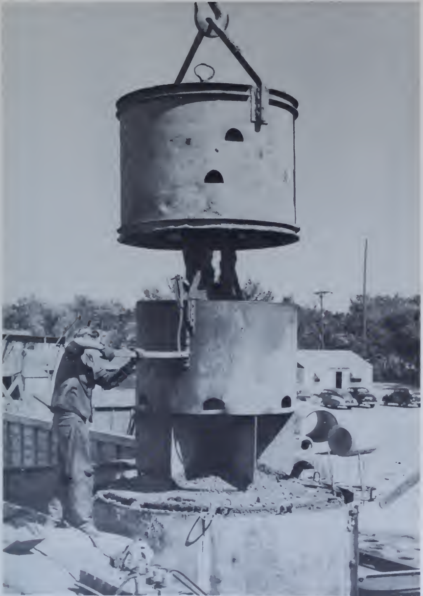
Figure 161.—Concrete placement by slow uniform flow over a conical surface. Manual operation of the butterfly valve at the outlet of the placing bucket and continuous vibration are used to control flow. The bucket at the top of this photograph is used for transporting concrete to the placing bucket. PX-D-33526.
